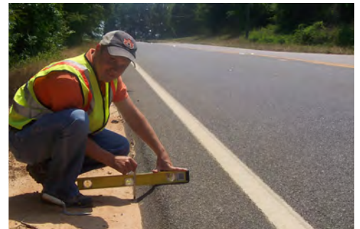
Example of the SafetyEdge SM after backfill material settles or erodes. Source: FHWA
